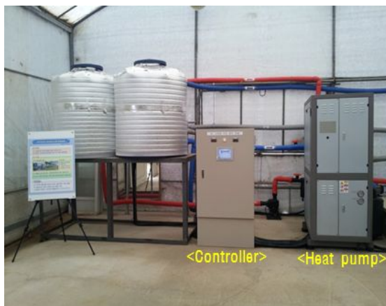
Fig. 2 System installation view
